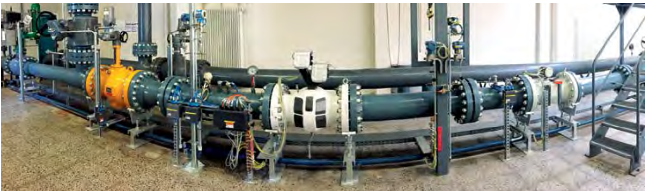
Pressure regulation station with the FLOWSIC600-XT Quatro and FLOWSIC600 at terranets bw.
